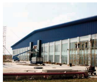
TBC-Ball Beverage Can (Vietnam) Limited under construction. Expected completion by second quarter of 2012.
