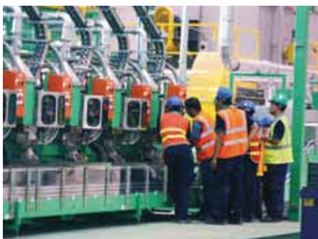
Engineering team conducted trial run after installation of the machines at TBC - Ball Beverage Can Vietnam Ltd.
